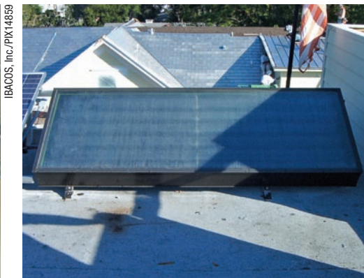
A solar thermal hot water system preheats incoming water.
