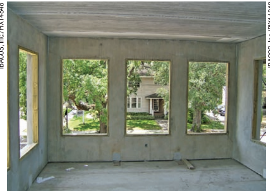
Openings for windows and any other penetrations required careful design and placement in the pre-cast concrete system.
