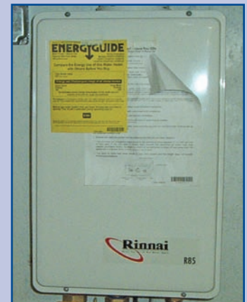
High efficiency water heaters save heating energy, while still providing ample amounts of hot water.
