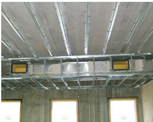
Well-sealed, fiberglass ductboard is completely enclosed in conditioned space.
