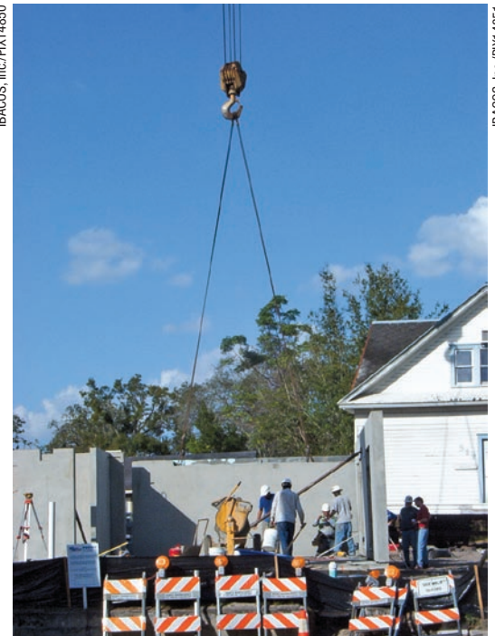
Pre-cast exterior concrete walls allow for faster building enclosure construction and a tighter envelope.
