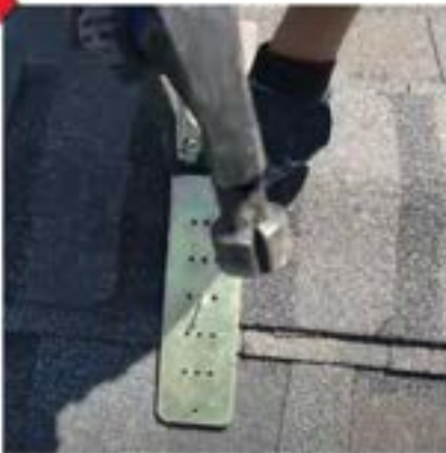
NAILS AND SCREWS DAMAGE ROOFS
