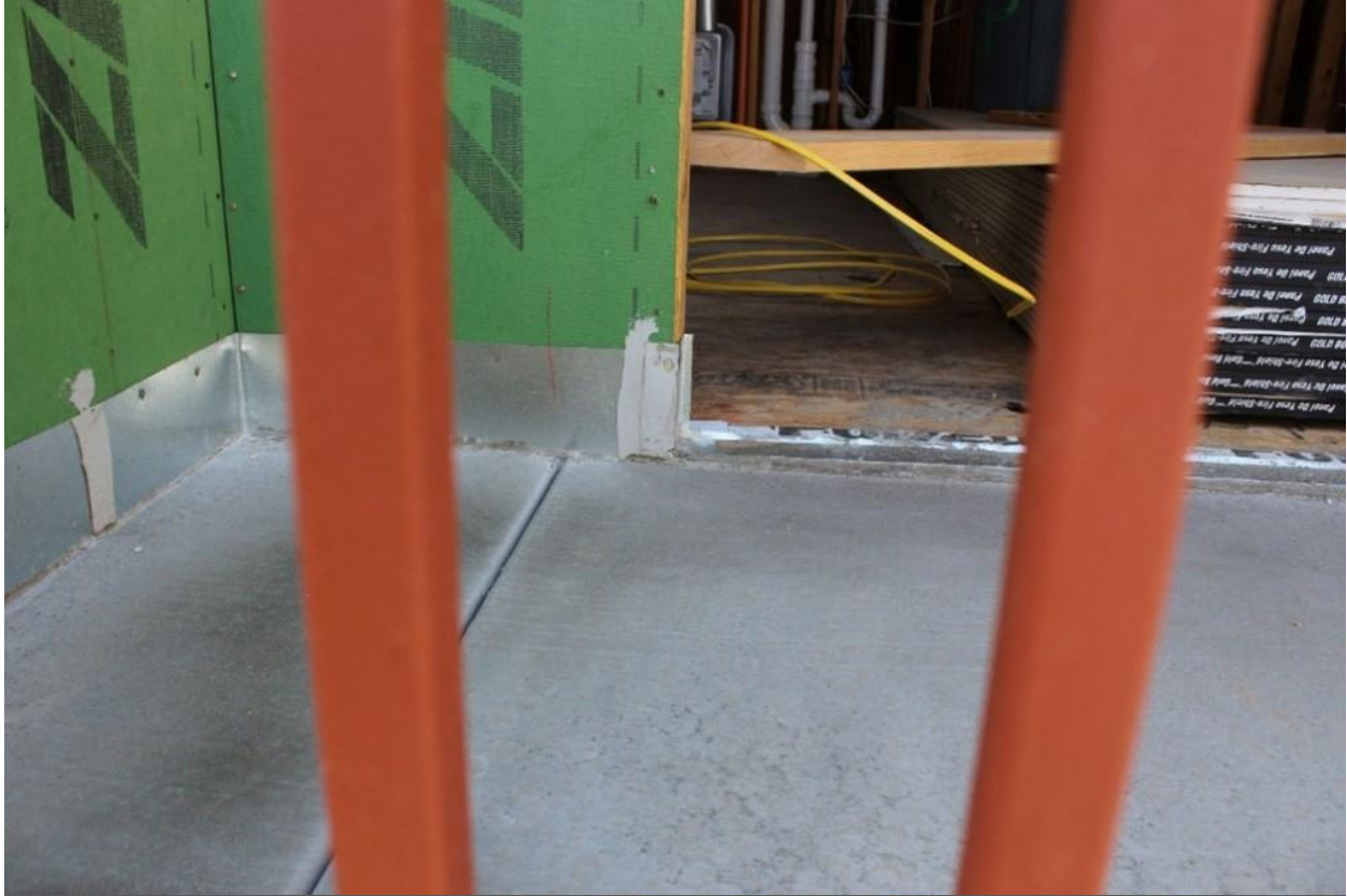
Deck to wall flashing installed over the ZIP System panels creating a reverse lap.
