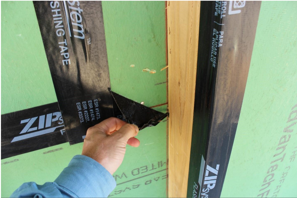
ZIP System Tape was not adhered near the end of a seam at an inside corner.
